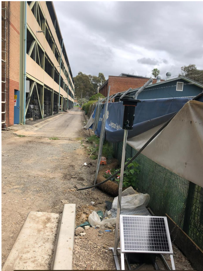
Figure 6 – Location 1 noise and dust monitor installation (SiteHive Hexanode 000108)
