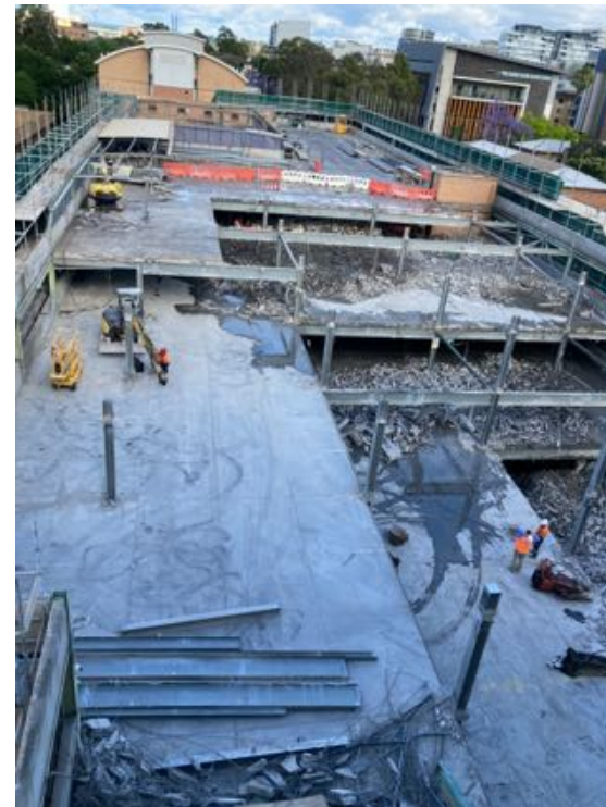
Photo 4 – General view of the demolition area. Works in progress within a well-enclosed area.
