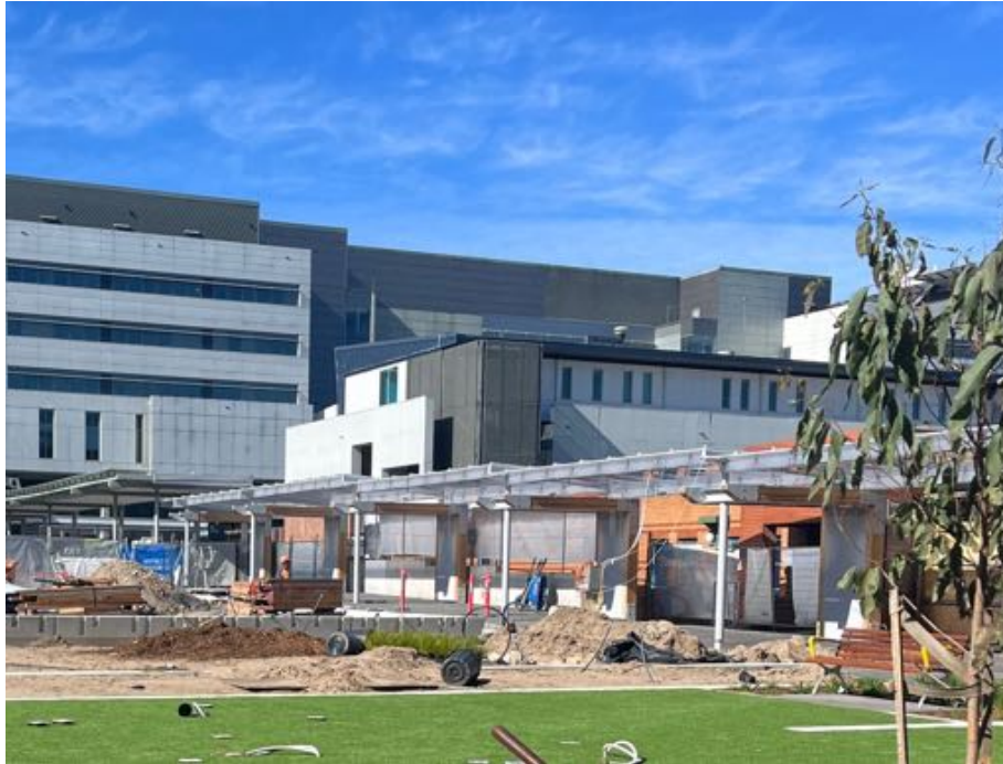
Photo 9 – Walkway to the new car park complete and soon to be handed over. Fencing will be moved to enclose the landscaping works area.
