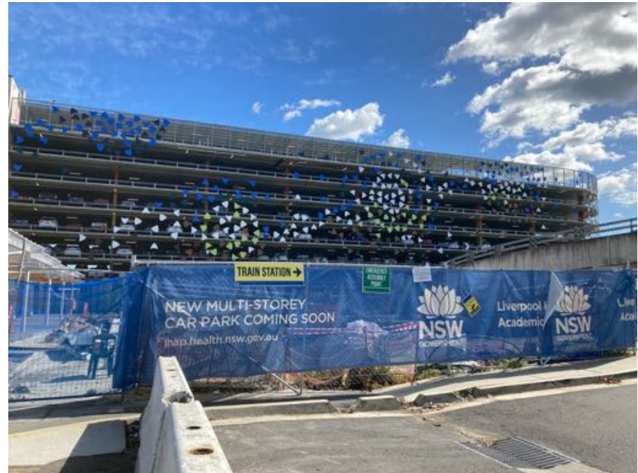
Photo 12 – Fencing around the landscaping works area. Operational multi storey car park in the background.
