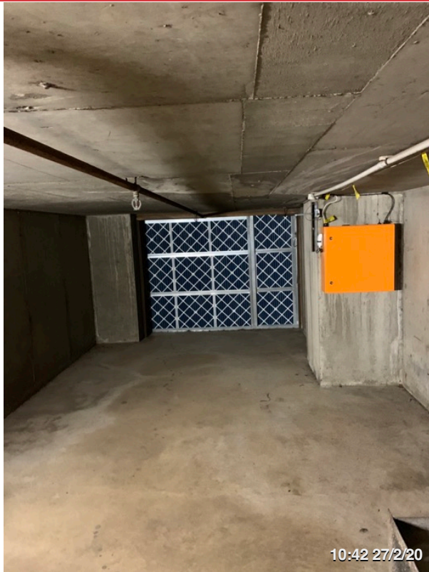
Building B Outside Air
