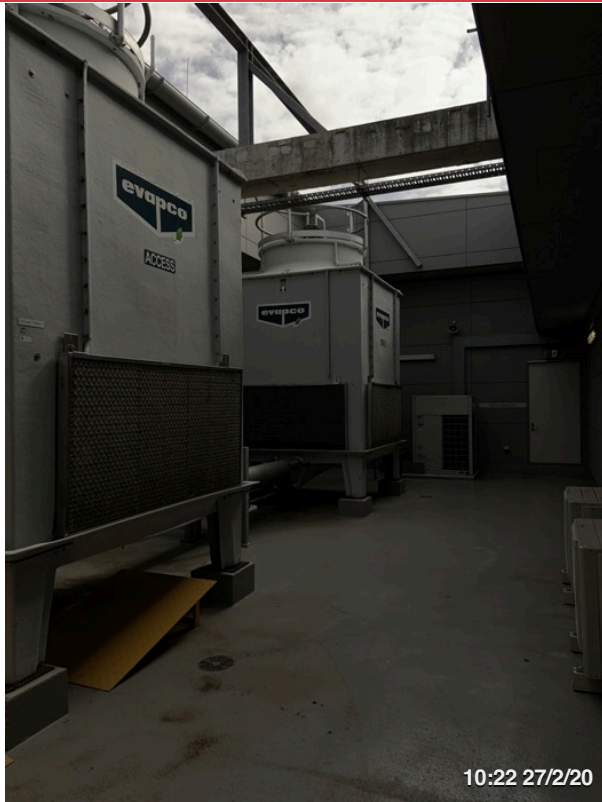
Cooling Tower Area
