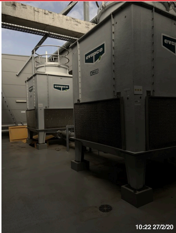
Cooling Tower Area
