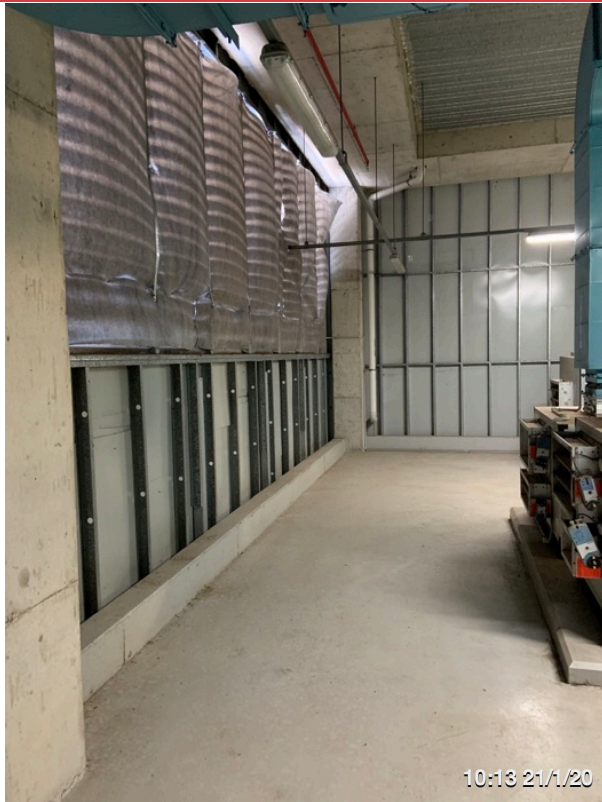
WESTERN PLANTROOM OUTSIDE AIR
