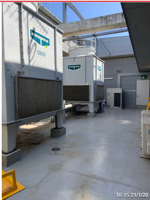
COOLING TOWER AREA
