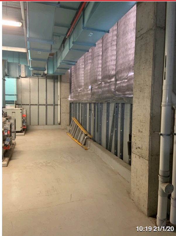
EASTERN PLANTROOM OUTSIDE AIR
