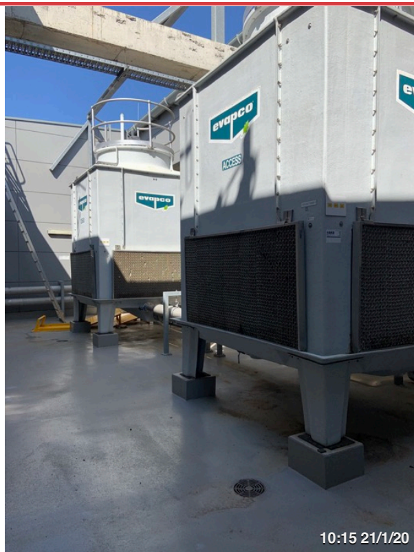
COOLING TOWER AREA
