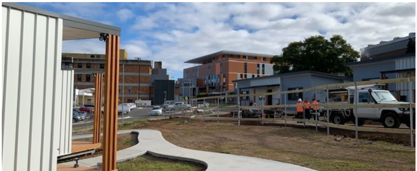
Several of the new units in place, with landscaping and fencing to be completed
