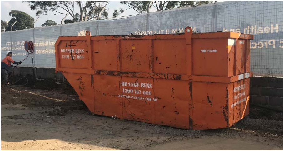
Photo 7 – Waste bins were available and empty.
