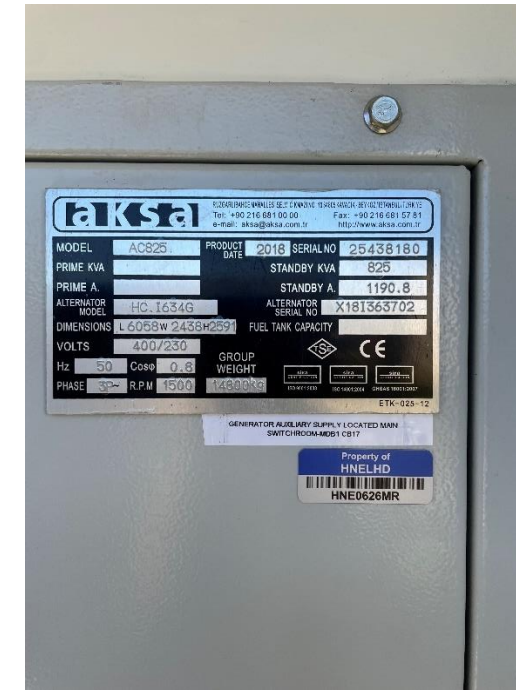
Figure 4-6: The Existing Generator Rating
