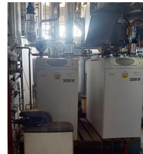
Figure 3-3: Existing Heating Hot Water Plant
