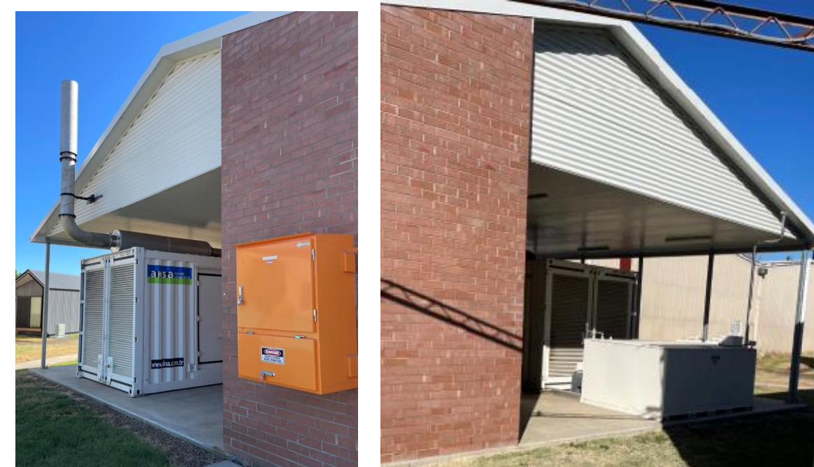
Figure 4-7: Containerised Generator and Link Box (Left)- Fuel Tank (Right)
