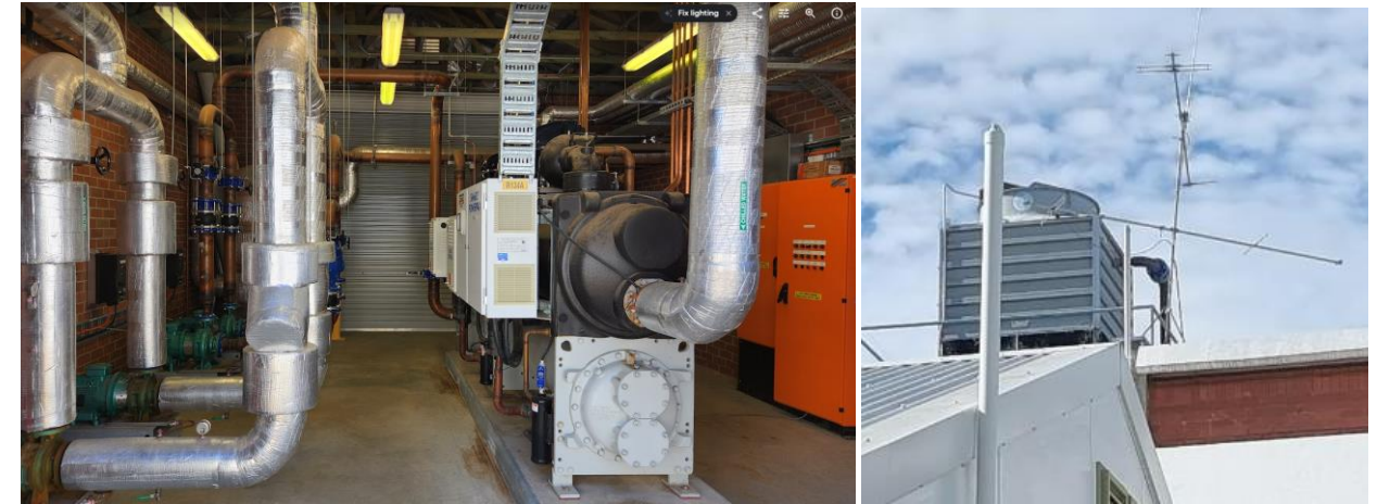
Figure 3-2: Existing Chiller & CT Plant
