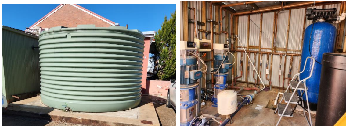
Figure 5-4: Photo of break tank, water softener, booster pumps and manifold
