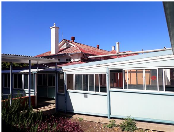
3 View south showing the northern wing and fibro covered walkways crowding the building.
