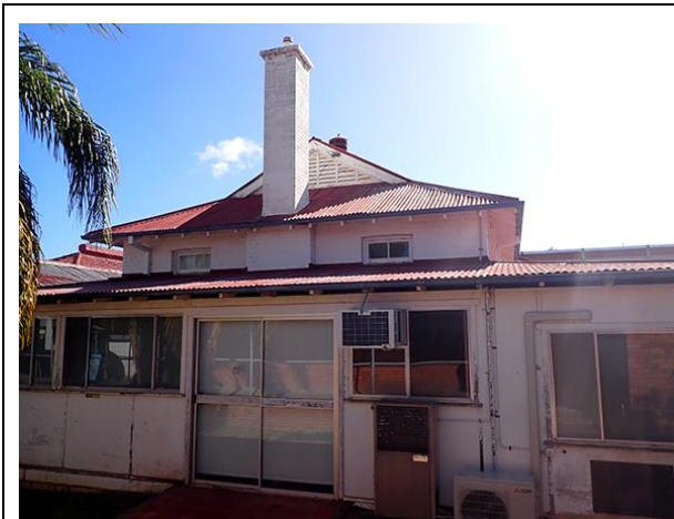
1 View north showing the southern façade of the building (under the higher roofline) and the unsympathetic fibro additions.
