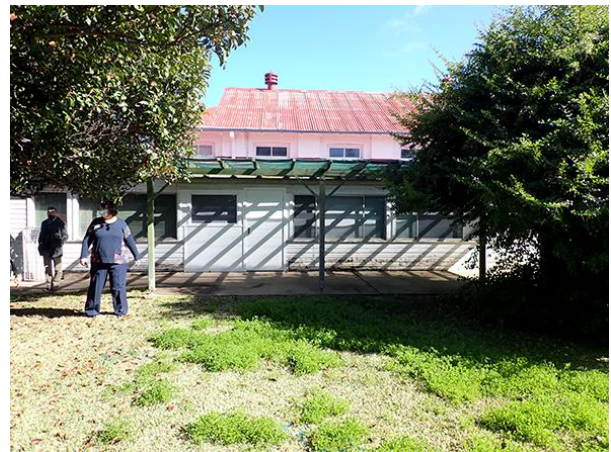
2 View west showing the southern wing with both a fibro addition and timber awning extending east.
