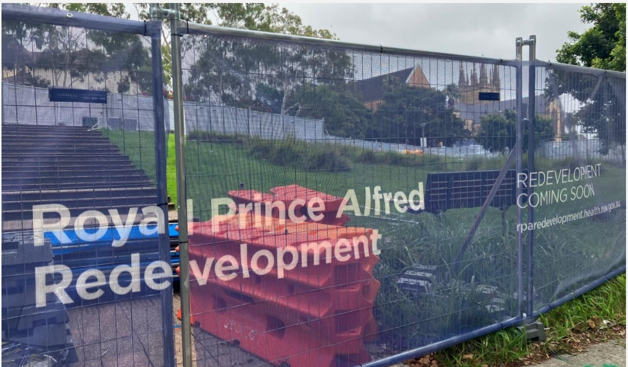
Site established for sewer main diversion/connection and temporary booster relocation on Lambie Dew Drive and John Hopkins Drive.
