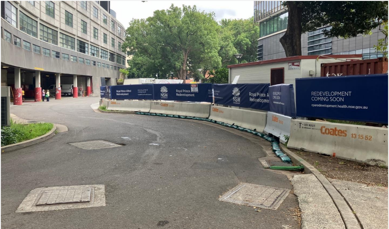
Lambie Dew Drive. Jersey barriers with shade cloth and sandbags installed. Requirement for loading dock at Clinical Services Building to remain clear at all times. Future OOHW will occur in this area to retain day time access to loading dock.
