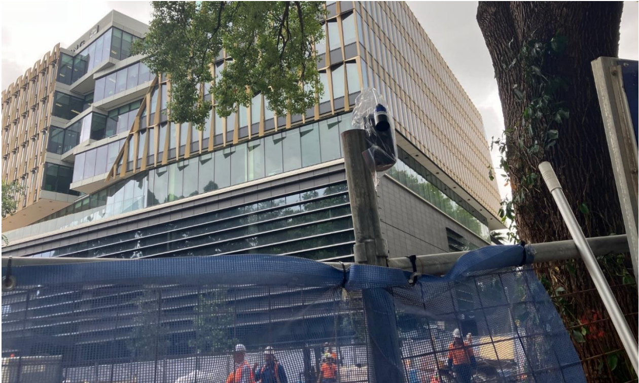
Air quality monitor installed for demolition works. Monitoring results and clearance certificates available on the project website.
