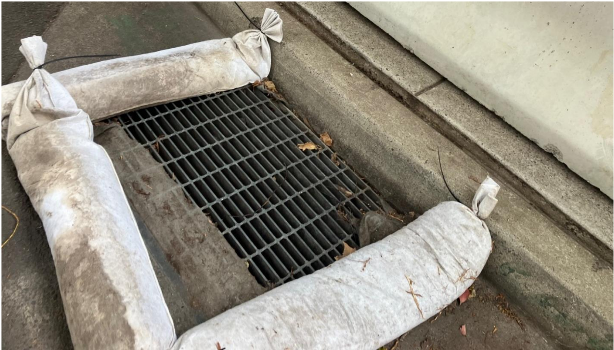
Pit drain protection throughout the site
