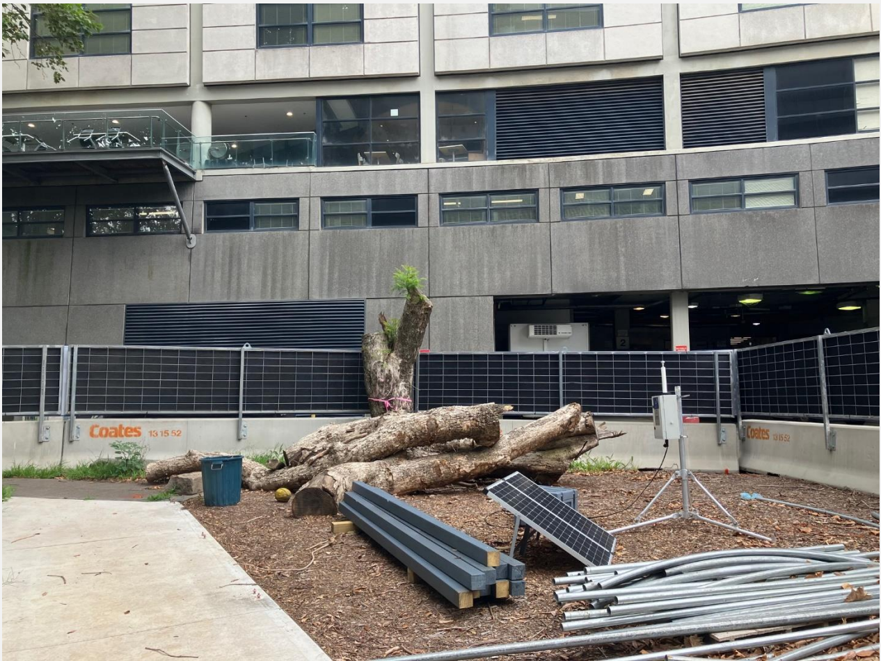
Removed trees at demolition site which will be reused at a later stage of the project.
