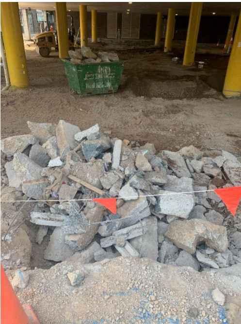
Concrete waste, surplus contained to designated area awaiting concrete waste bin servicing (emptying)
