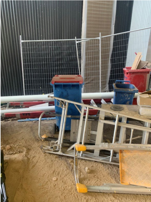
Poor housekeeping, materials stockpiled in front of bins, bin waste streams not evident, discarded materials (poly-pipe) with equipment (ladders)
