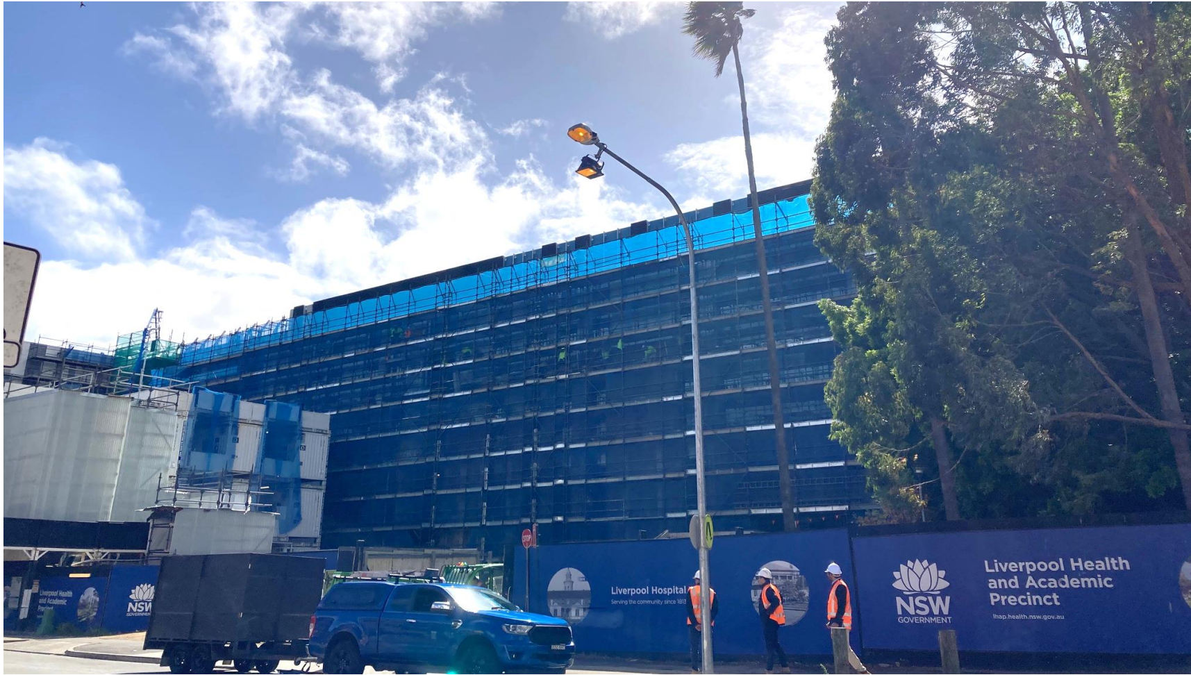
Photo 13 – View of the site on Goulburn Street. Structure being completed, hoarding around the perimeter of the site, tree protection for trees on the corner with Elizabeth Street.
