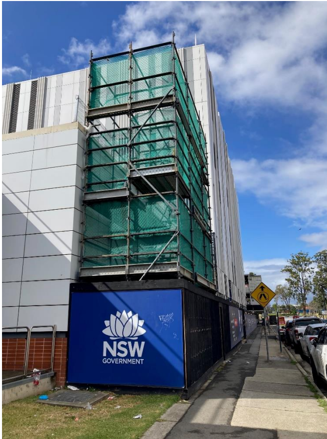
Photo 3 – Hoardings in place on Goulburn Street around newly built structure. Footpath clear of obstacles.
