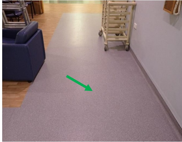
Photo 2: Level 1 Gait lab, staff kitchen area, top of floor – Non-asbestos blue vinyl flooring
