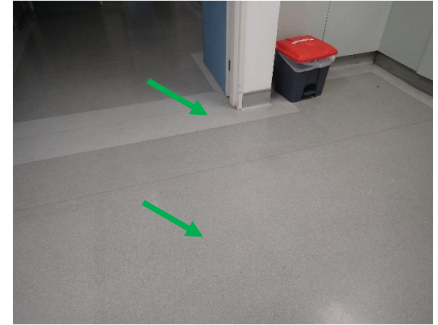
Photo 15: Level 2 Old Emergency Department, throughout emergency department, flooring – grey and light grey non-asbestos vinyl flooring
