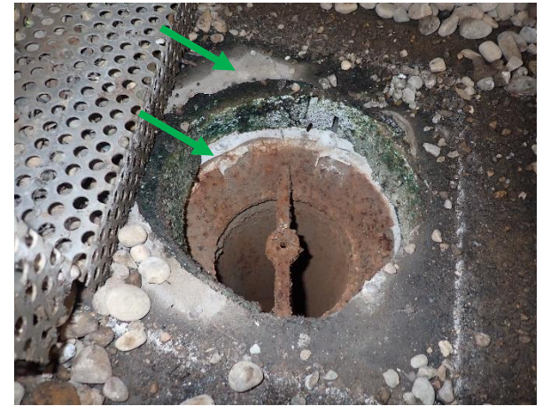
Photo 27: Level 2 Pathology Expansion Area, northern courtyard portion, flooring – non-asbestos fibre cement. Non-asbestos waterproofing material observed
