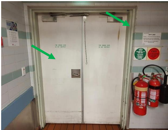
Photo 10: Level 1 Kitchen, north entry fire doors – assumed non-asbestos fire doors as doors were identified to be manufactured in 1990's or 2000's. Non-lead based light green paint on door frames
