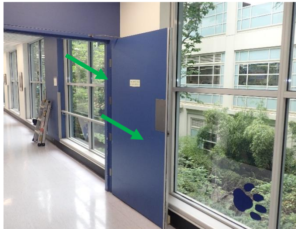
Photo 23: Level 2 Linkway and Pathway, fire doors and door jambs – Non-lead based blue paint. Fire doors observed to be manufactured in 1990s and is assumed to not contain asbestos
