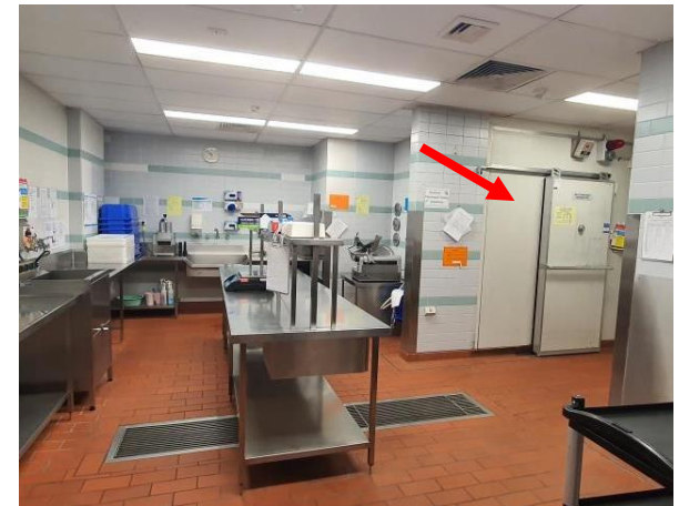
Photo 12: Level 1 Kitchen, north area of kitchen – cool rooms assumed to contain internal SMF insulation
