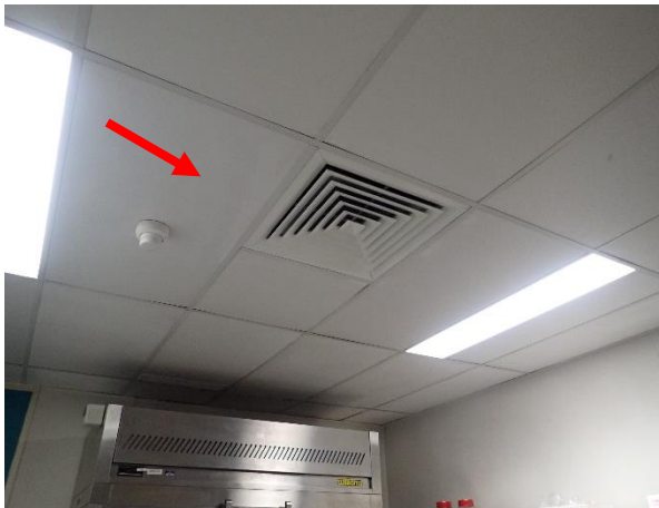
Photo 4: Level 1 Gait lab, kitchen, false ceilings throughout – false ceiling tiles assumed to contain SMF
