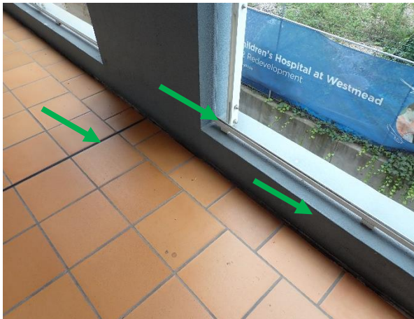
Photo 22: Level 2 Linkway and Pathway, external area, glass balustrade and between tile flooring – non-asbestos black mastic sealant.
