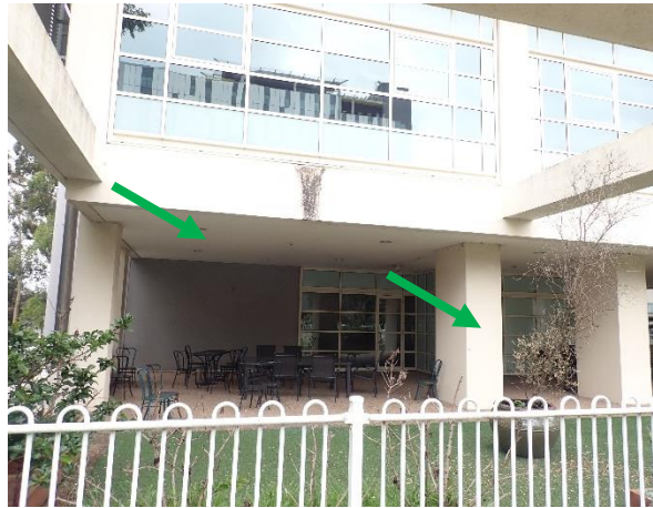
Photo 26: Level 2 Pathology Expansion area, external area, soffit lining – non-asbestos fibre cement. Non-lead based white paint on concrete pillars
