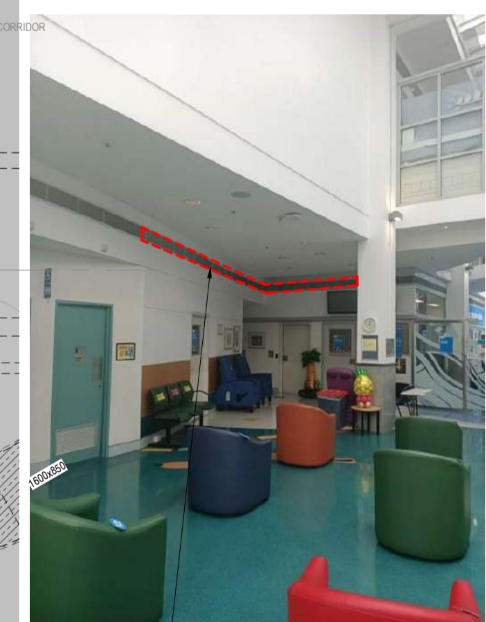
EXISTING LINEAR GRILLE SERVING THE GALLERIA TO BE DEMOLISHED AND STORED ON SITE FOR INSTALLATION IN NEW CEILING LINE
