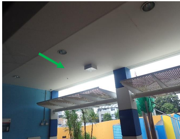
Photo 17: Level 2 Old Emergency Department - external smurf garden, soffit lining – non-asbestos fibre cement
