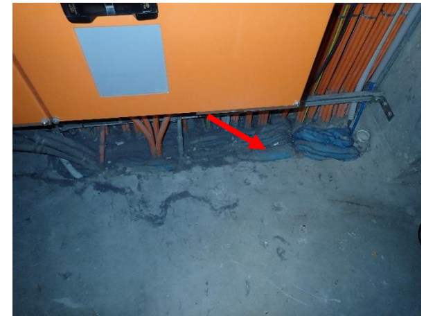
Photo 24: Level 2, Linkway and Pathway, electrical cupboard, cable penetrations – insulation pillows assumed to contain SMF
