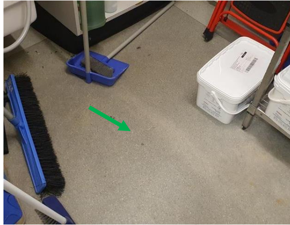
Photo 8: Level 1 Kitchen, chemical storage room, top of floor – non-asbestos grey vinyl flooring
