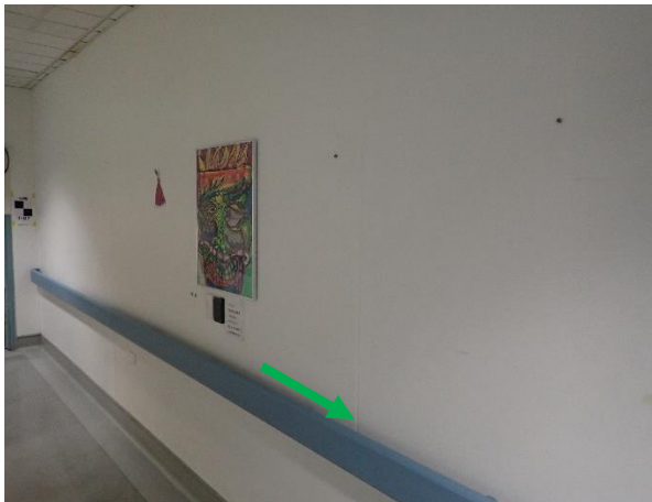
Photo 16: Level 2 Old Emergency Department - cement rendered walls, between walls – non-asbestos expansion joint
