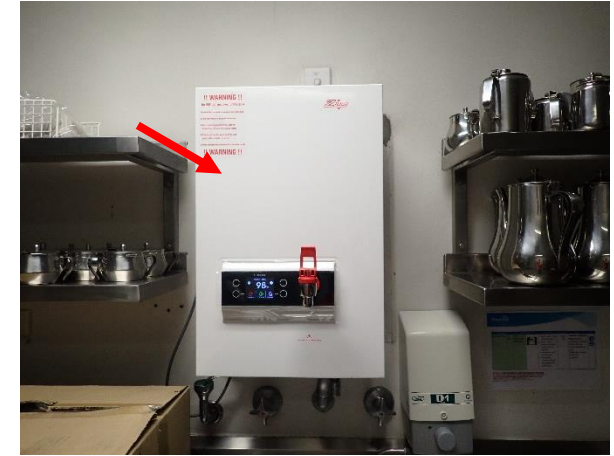
Photo 3: Level 1 Gait lab, staff kitchen and meeting room – hot water unit assumed to contain internal SMF insulation
